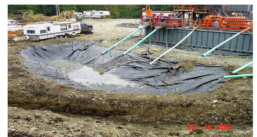
A waste pond is man made; it is used to dispose of contaminated waters created as a result of natural gas and other types of drilling.
